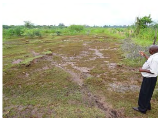
Photo 2.1.2 Broken Point of the Embankment Canal-C
