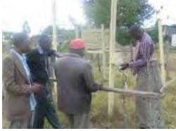
Installed rain gauge for CBFWS
