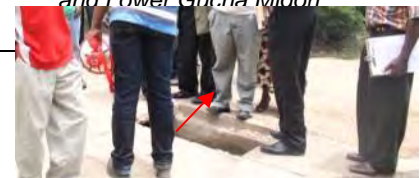
Vandalized culvert slab pavement
