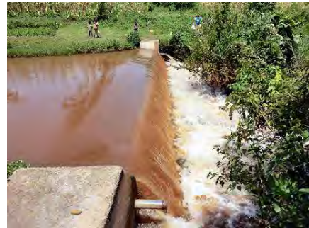
Check Dam (Example of Nzoia River)
