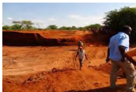
Washout of the concrete bridge of the same structure to the above by flash flood Place : Rengesa
