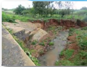
River Bank erosion before bank Protection
