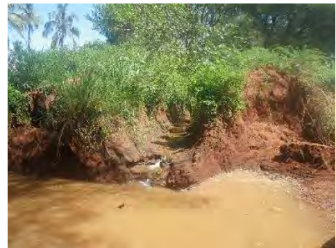
Irrigation canal broken down by flash flood from lateral face
