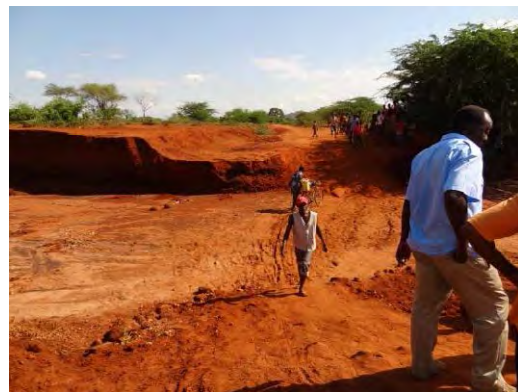
Road Bridge rushed out Place : Rengesa
