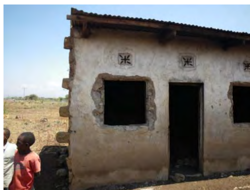
House was destroyed by flood
