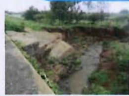
River Bank erosion before bank Protection
