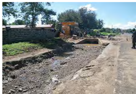
Very few drain channel installed in the urban area Place: Isiolo Town
