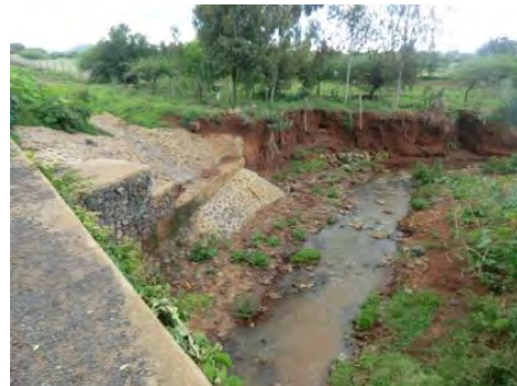
Bank erosion at the Eastern Marania River
