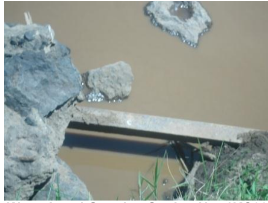
Water Level Gauging Station No.:1KC03 Observation River: Migori River Special Note: Water level gauge is broken off and damaged.
