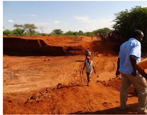
Road Bridge rushed out Place : Rengesa
