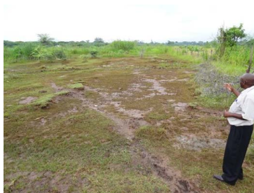
Photo 3.1.2 Broken point of the embankment Canal-C
