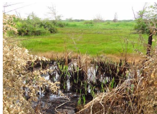
Damp ground where the bank of Canal-C has been washed out
