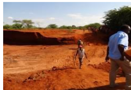
Washout of the concrete bridge of the same structure to the above by flash flood Place : Rengesa
