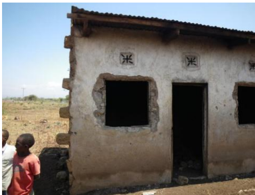
House was destroyed by flood
