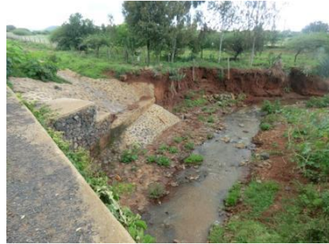
Bank erosion at the Eastern Marania River
