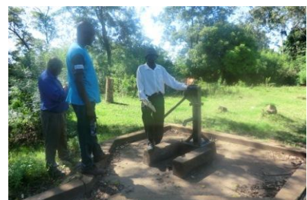
Water point at former Kabuto School, the borehole is currently damaged
