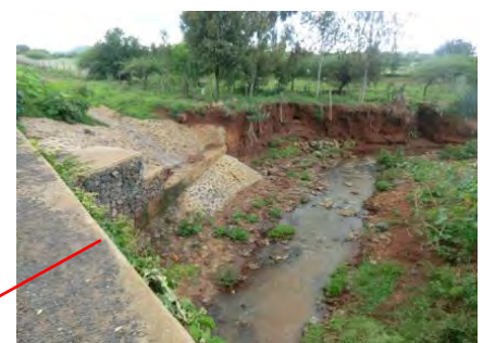
Eroded bank before protection
