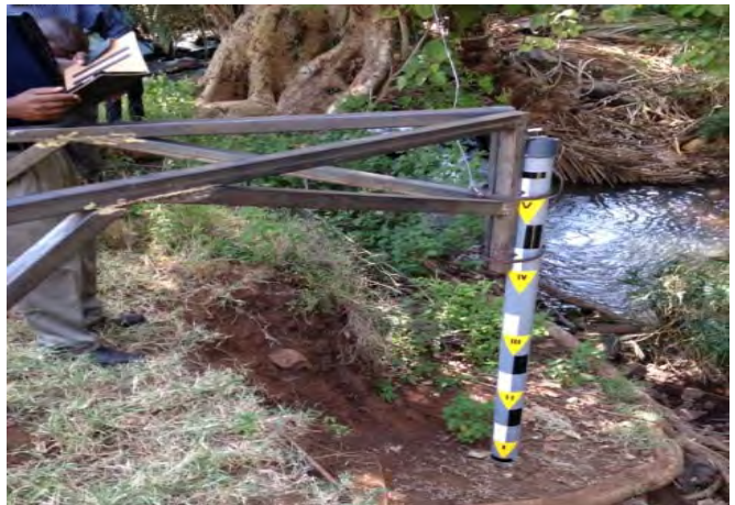
Installation on a metal fabricated stand (Kenya)
