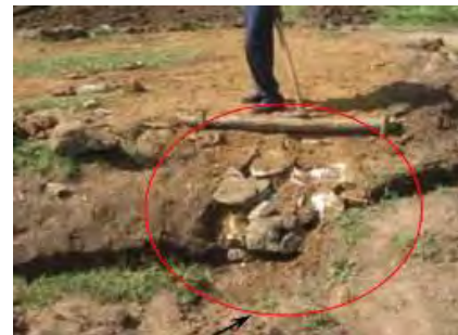
Protect the entry and exit walls from clogging due to erosion
