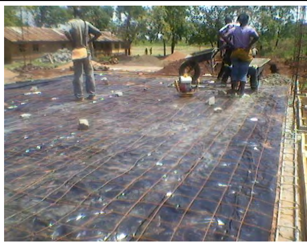
Date: 20-01-2014 Description: Preparation for foundation the floor slab, BRC 142 and DPC Polyethylene sheeting
