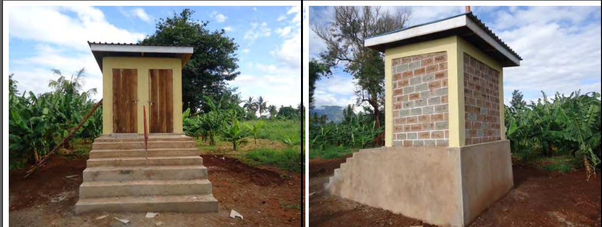
Date :07-04-2014 Description : Finished Toilet front view Date :07-04-2014 Description : Finished Toilet side view
