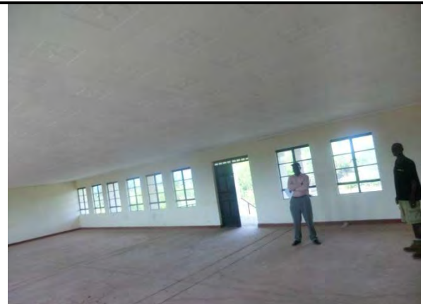
Description : Well-maintained EVC that hosted at least 200 flood affected persons in the last flood occurrence
