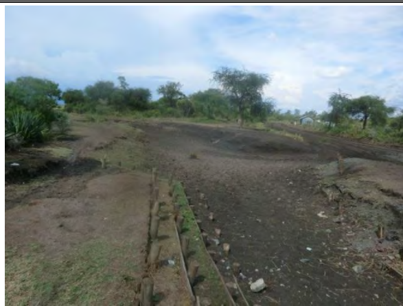
Description : Weir is silted and community members have not remove the silt inspite of the dry season leading to overflow of water
