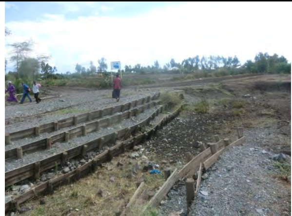
Description : Poorly maintained weir with some wood planks having been vandalized
