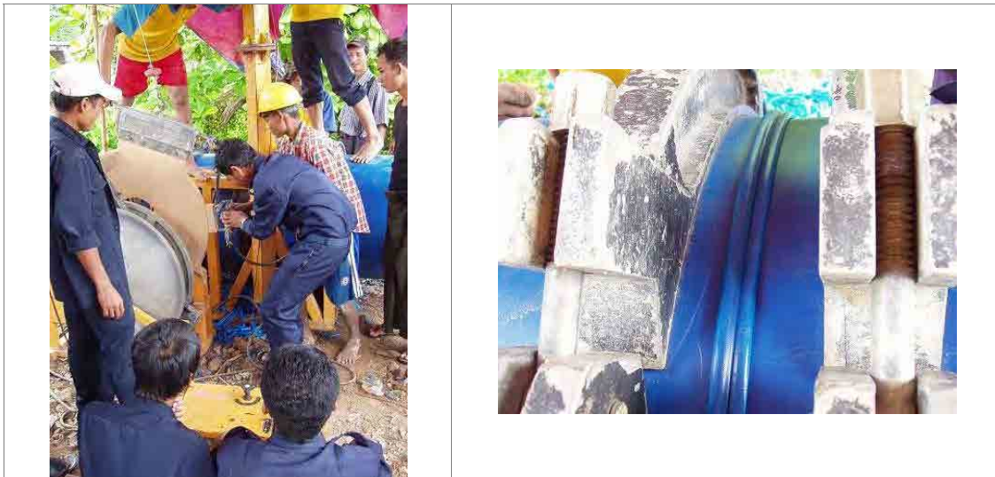
Photo 5.2 A Field Training of \phi 800 HDPE Pipe in Plumbing of Large Pipe Course
