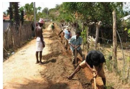
Construction of a water supply system by CMR. The community members provided labour free of charge for excavation and backfilling of pipe laying (Velloor village in June 2009)
