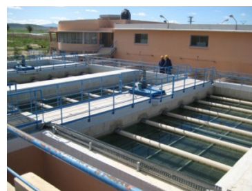
Oujda Water Purification Plant
