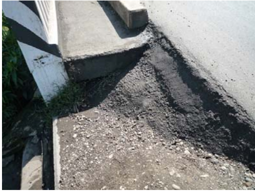
After the asphalt overlay on the approach bridge (Soil was settled to the degree shown above)
