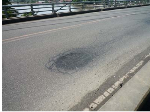
Pothole on the bridge carriageway (repaired)
