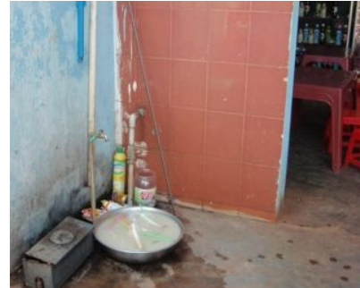
Water faucet and meter box at a café / house. After the introduction of tap water, the family stopped using the dug well since it was located close to the toilet. Now, tap water is used for household use, glass washing at the café, and hand washing by café customers.
