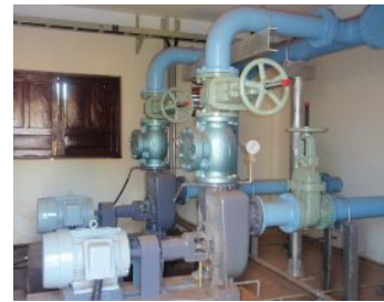
Distribution pump (Nhon Hoa)
