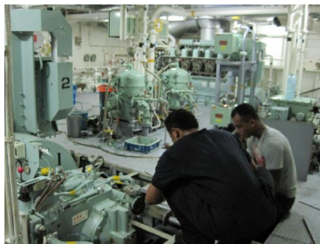
Photo 7: Inspection of the main engine
