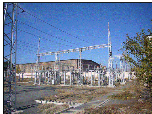
Rehabilitated Echmiatsin Substation
