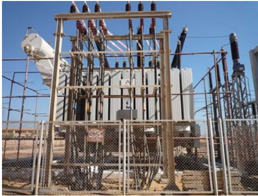
Substation installed by the project
