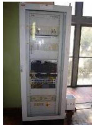
SCADA-related Facility in Yerevan Power Plant
