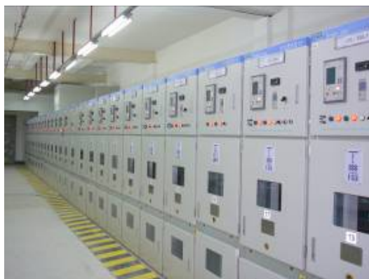
Instrument rehabilitated at Kirza Substation
