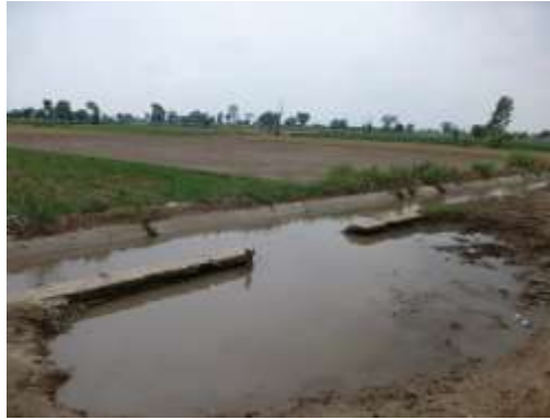
Chart 9. An example of a leaking minor
