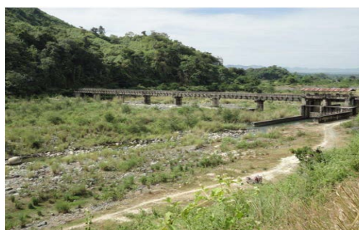
NIA irrigation intake
