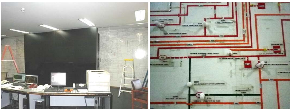
Distribution Control Room (left; large display units not in use, right; manual display unit)
