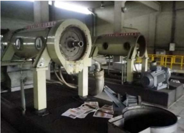
Sludge Centrifugal Dewatering Units (Penha WWTP)
