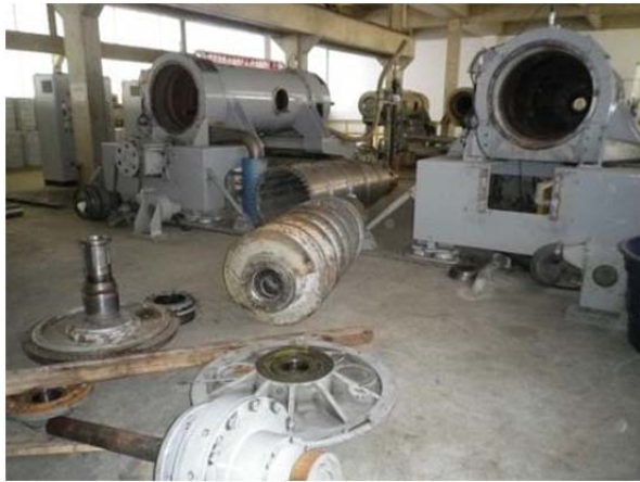
Sludge Centrifugal Dewatering Units waiting for repair (Alegria WWTP)
