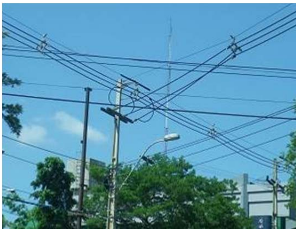
23kV distribution lines
