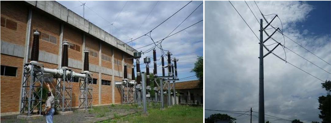
Parque Caballero Substation (the facility not yet connected)
