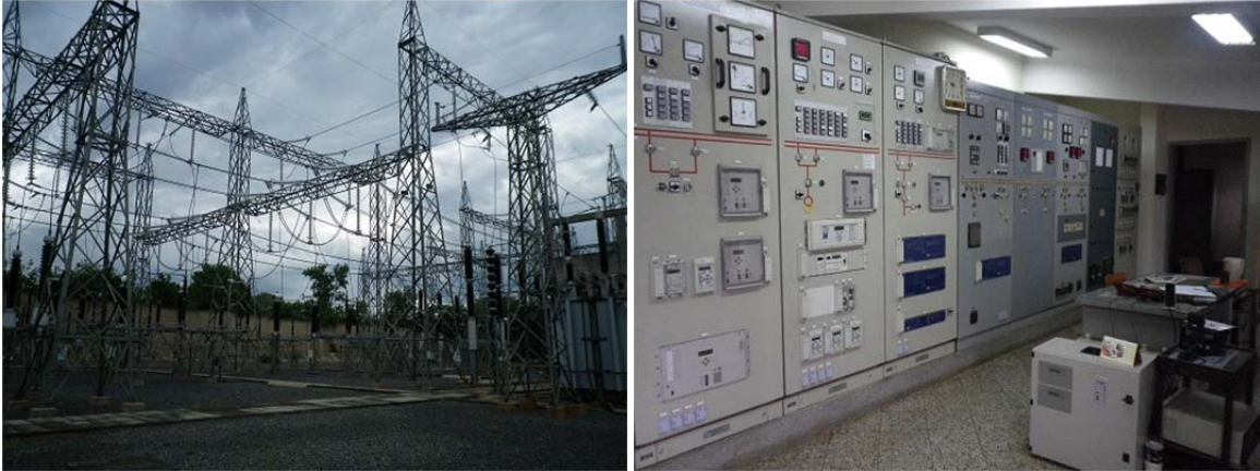
Puerto Sajonia Substation (left; switch yard, right; control room)
