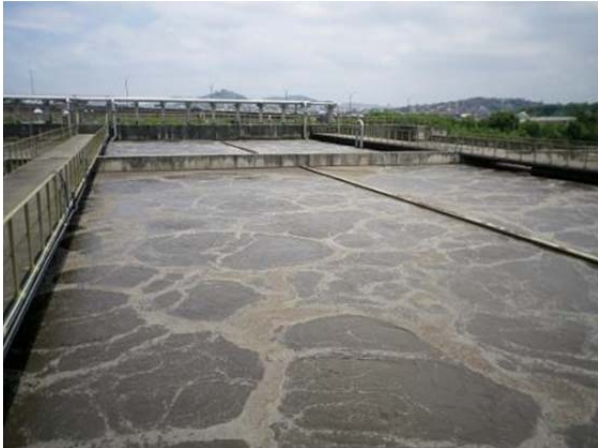
Secondary Treatment Facility (Alegria WWTP)
