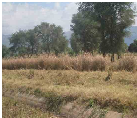
Picture 2: Grasses planted along the main canal, which the farmers' cooperative implemented for the protection of the bank from flood damages
