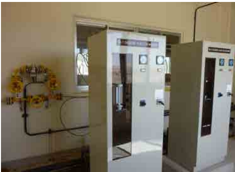
Photo 6: Procured and Installed Chlorination Equipment (Khaw Pumping Station)
