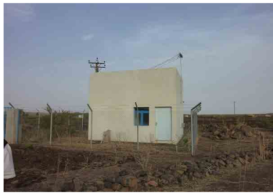
Figure 12: Well and Pumping Facility in Debarwa (it gets flooded in the case of heavy rain as the foundation and the door are built at too low an elevation)
