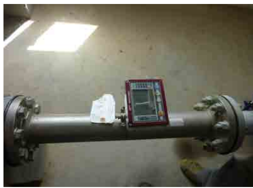
Figure 2: Non-Operating Flowmeter (Dekemhare)
