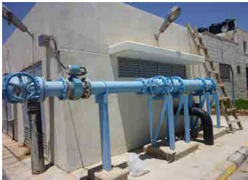
Photo 5: Renewed Pumping Facility (Batrawi Pumping Station)
