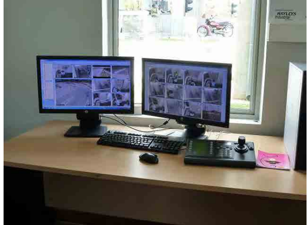
CCTV Monitoring System in Toll Office
