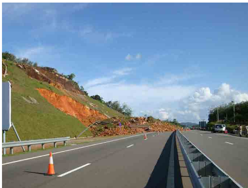
Photo 2-2-1 Land Slide Site at SEW42.5km East side (whole lanes for Galle direction and one lane for Colonbo direction was closed in Nov. 2012)
