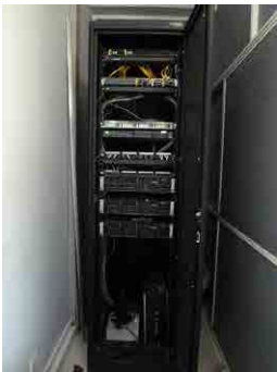
Existing Servers in Traffic Control Center
