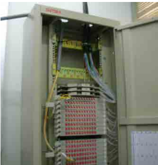
Cable Rack for Existing Optical Fiber Cable
