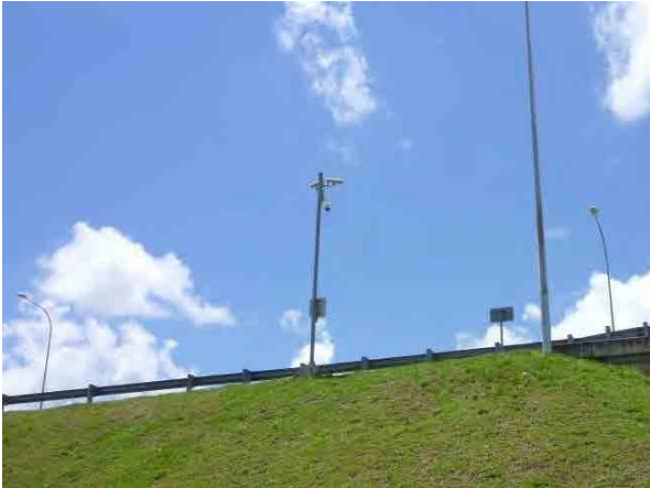
Existing CCTV Camera
