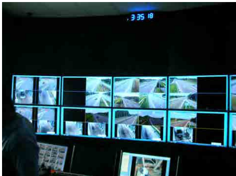
Monitors in GelanigamaTraffic Control Room
