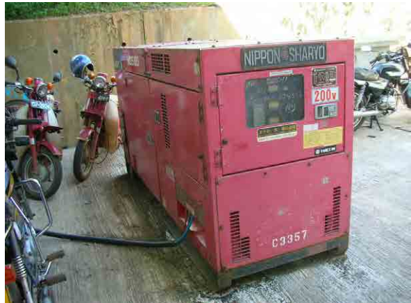
Back up Engine Generator in Toll Office (Temporary Equipment)
