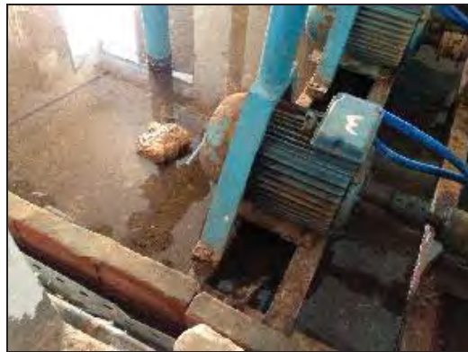
Inundated pumping station (Medenine)
