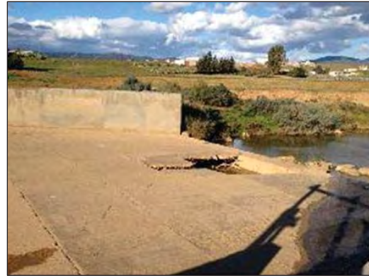
Crack in the threshold of rainwater pumping station (Fernana)
