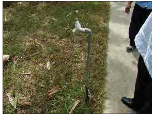
Faucet for Reused Water (Mactan)
