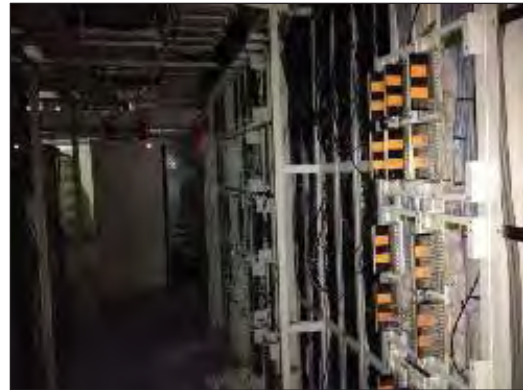
Switching Station (Harare)
