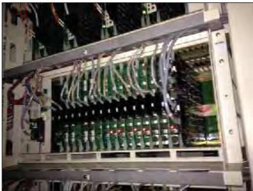
Switching board: empty slots can be seen
