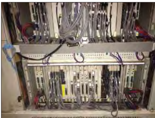
Switchboards: empty slots can be seen
