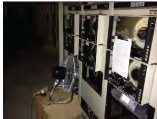
Fan is used to substitute for cooling system
