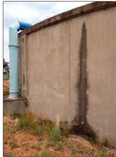
Ekangala Regulating Reservoir Minor leakage can be seen
