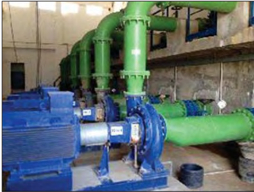
Pumping Station (Fernana)
