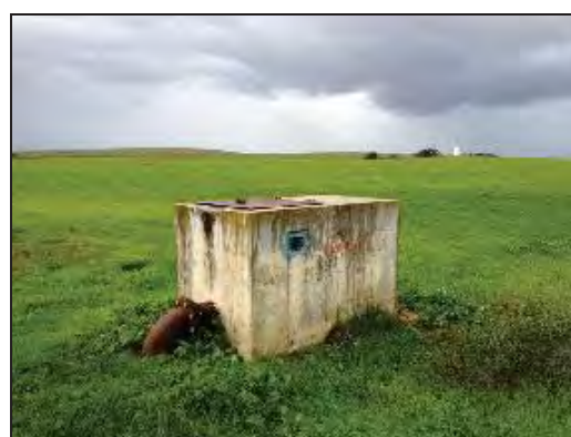
灌漑用の配水栓
