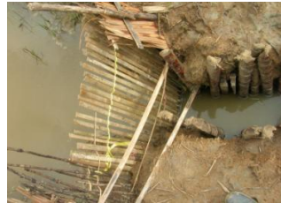
Bamboo Slates Gate: Bamboo slates are set up to inlet of the pond
