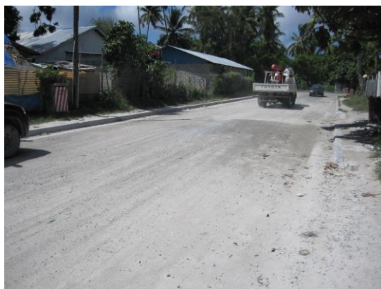
Photo 2: Project Road with the Surface Broken Away (Taatirerei Road)
