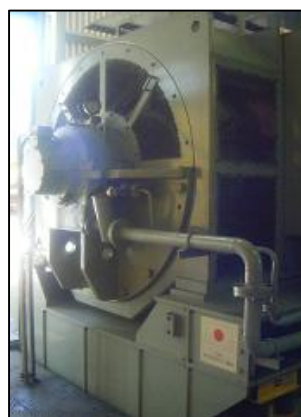
Installed Diesel Engine Generator
