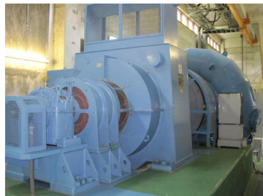
Generator Unit Provided in the Project
