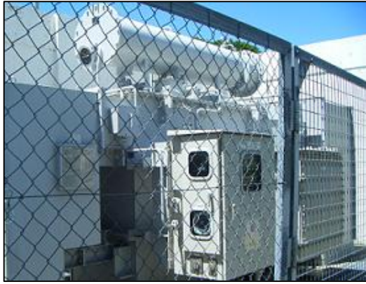
Transformer in Ranadi S/S
