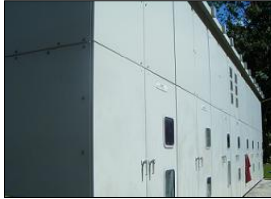
Switchgear in Honiara East S/S
