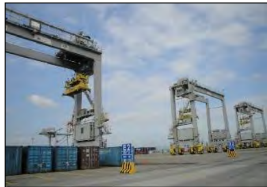
Rubber Tired Gantry Crane
