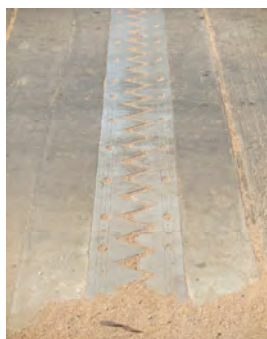
Sand clogging joints due to lack of cleaning
