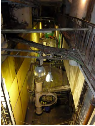
Water valves of all three units
