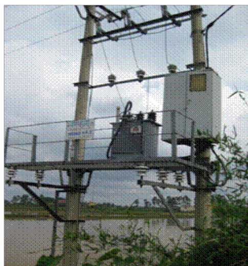
(A substation in Bac Ninh)
