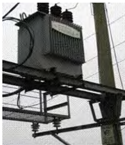
Pole mounted transformer made in Vietnam
