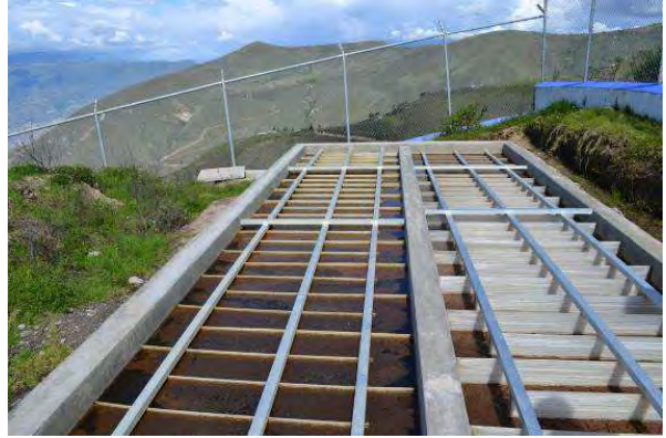
Rapid Filtration installed at Aloburo Purifying plant
