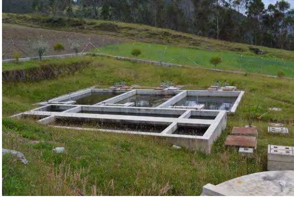
Purifying plant at Zuleta
