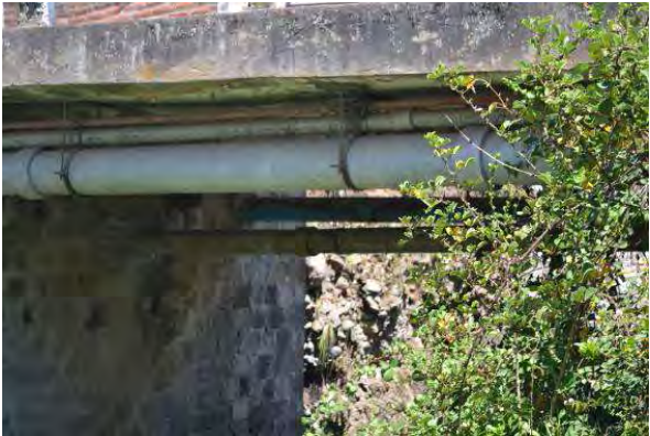
Conveyance pipe at Esperanza
