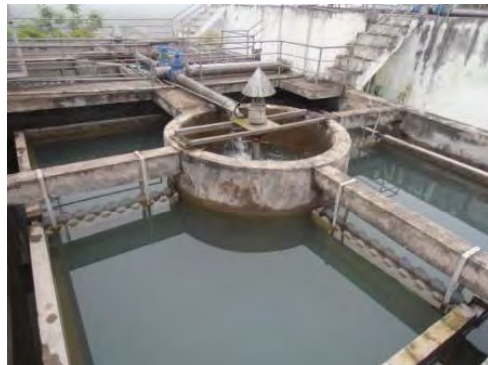
Filter basin in a treatment plant constructed by the project
