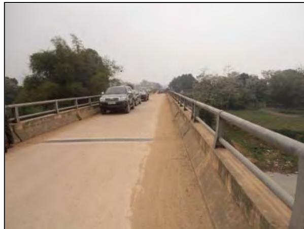
A bridge constructed by the project in Phu Tho province (Small boat was the only means of transportation before the project.)
