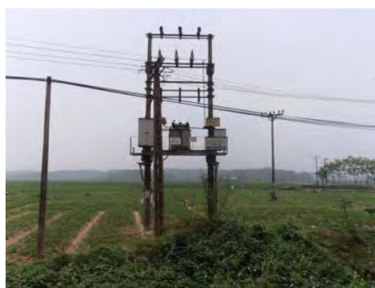
Distribution lines and transformer installed by the project
