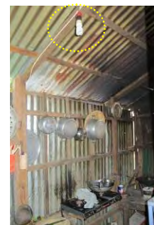
Lighting device installed in a kitchen
