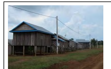
Power line in Laoka. Electricity is being provided to contracting households.
