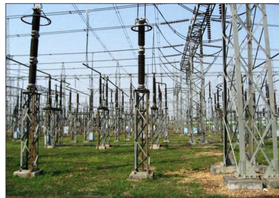
Overview of Equipment at Arambag 400 kV Substation
