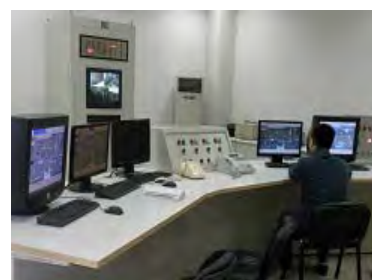
Central control room
