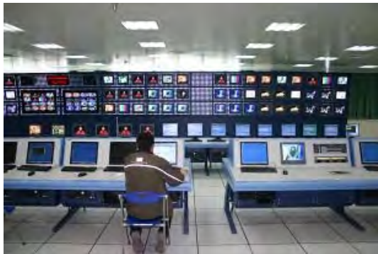
Jinan TV Station: monitoring room
