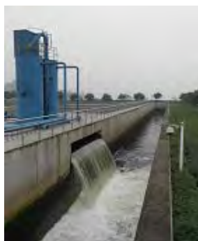
Wastewater Outlet of Juguanshi WWTP
