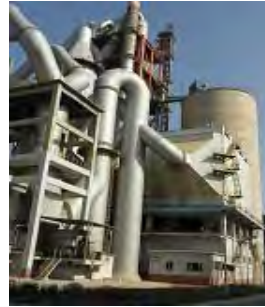
Dust remover installed at the tail of kiln
