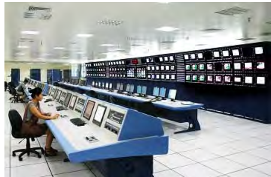
Jinan TV Station: monitoring room
