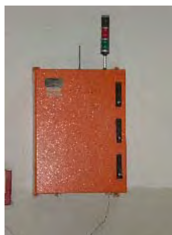
Network Equipment for Online monitoring system
