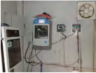
Wastewater monitoring equipment in Xinan Synthetic Pharmaceutical Factory
