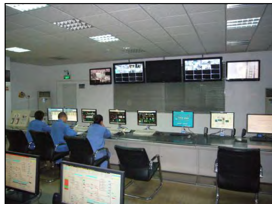
Blast Furnace Gas Combined Cycle Power Plant (Control Center)
