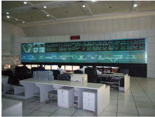
Train Operation Control Center
