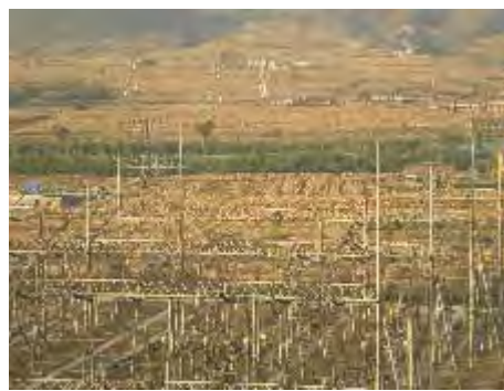
Transmission line from Wangue Power Plant to Shandong Province
