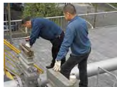
Staff inspecting the equipment at Toutong Station
