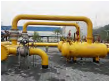
Filtration machine at Toutong Gas Storage Station
