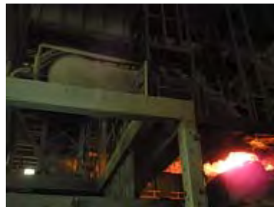
AOD furnace and dust remover
