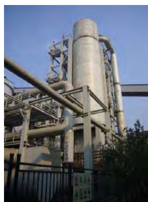
Desulphurization and HCN Removal Plant
