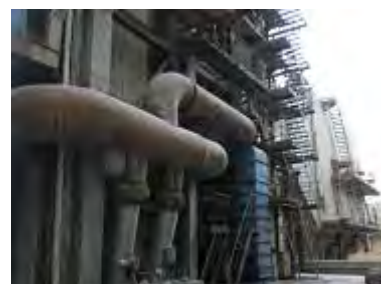
Exterior view of generation facility
