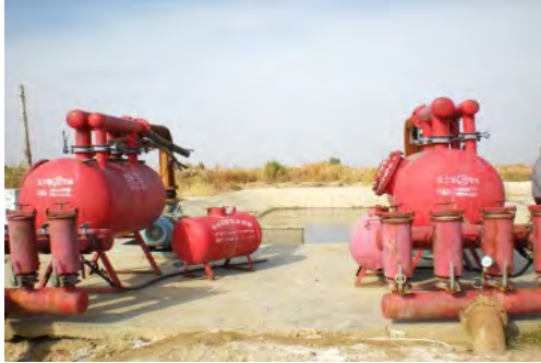
Pumping machine and fertilizer mixing machine (Tacheng)
