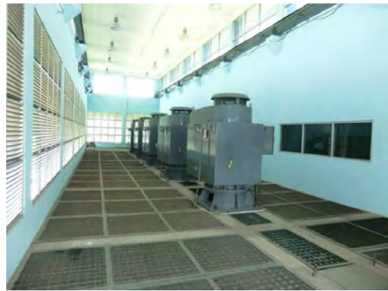
Photo 4 Water Supply: Wonocolo Pump Station
