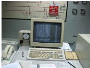
Picture 3 Monitoring Control System
