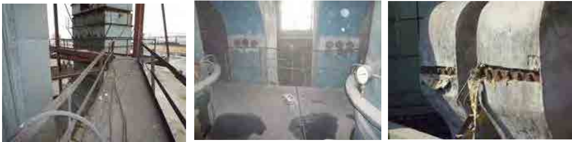
Fig. 3-6 Measurement Hole for Stack Gas Monitoring (PP4, PP3, PP2)
