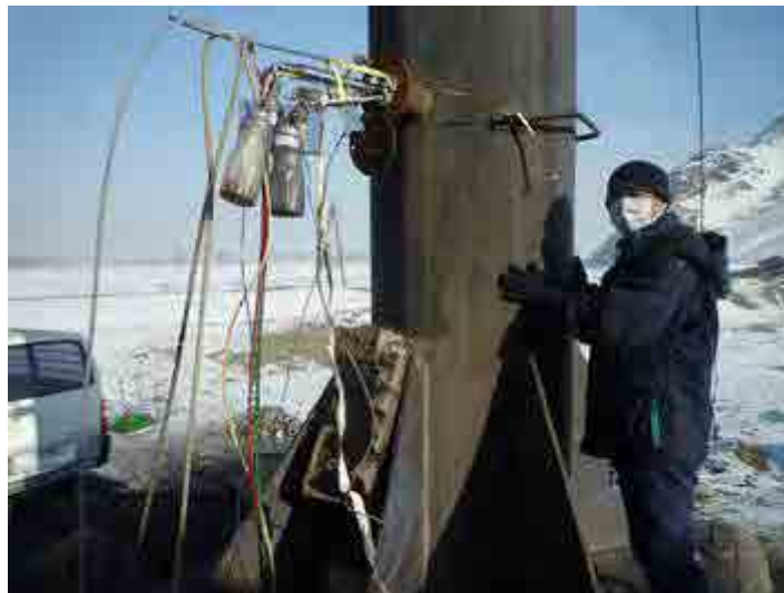
Figure 10-5 Installed Equipment on the Stack Side (For the Automated Equipment)
