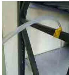
Incorrectly Fixed: The pipe gets squashed by its own weight where it is fixed.
