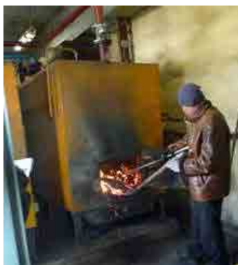
Fig. 3-1 Coal Feeding Work for HOB
