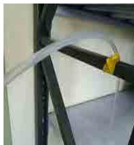
Incorrectly Fixed: The pipe gets squashed by its own weight where it is fixed.
