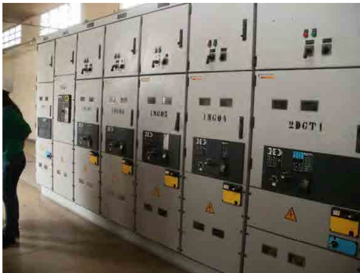
Fig. 4.3.3 MV Switchgear at Distribution Substation (AMPLA)
