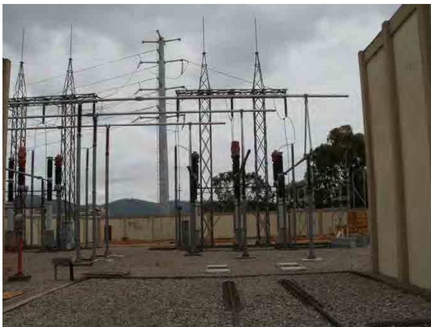
Fig. 4.3.2 Typical Distribution Substation (AMPLA)
