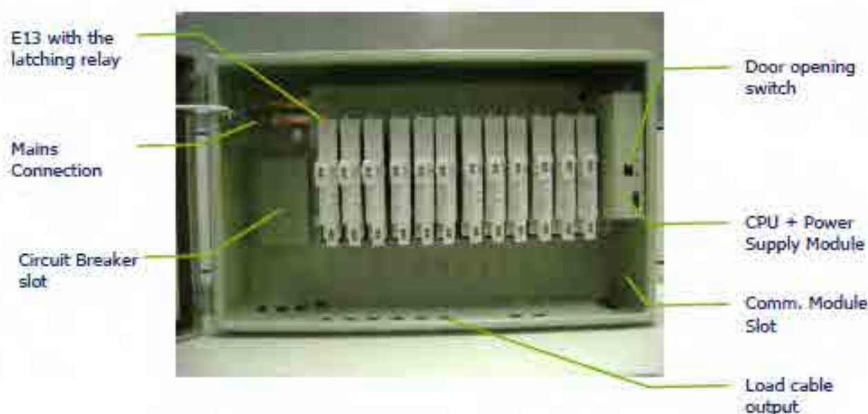
Fig. 4.6.3 An example of smart meter by Landis + Gyr (SGP+M)
