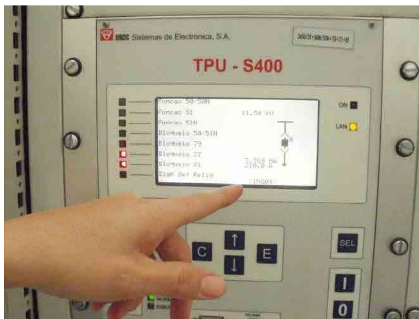
Fig. 4.3.4 Bay unit of 13.8kV Feeder
