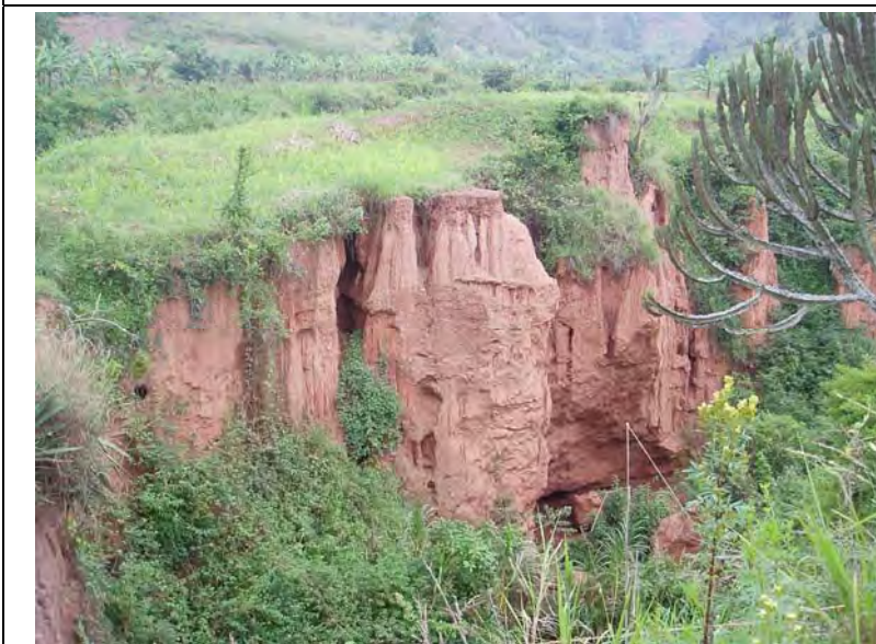
Gatsibo31 Gully near the dam axis. The depth about 15m, width about 15m.
