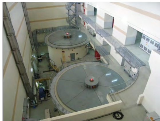
Photo 2: Hydropower plants with 300MW (150MW x 2)
