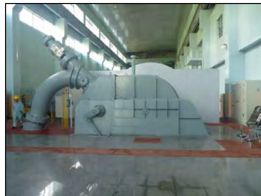
Da Nhim Power Station Turbine and Generator
