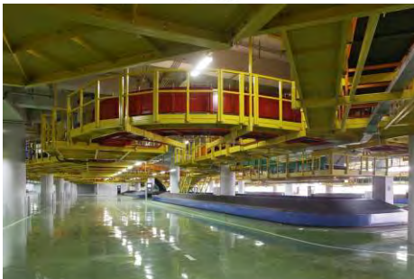
GF Baggage Handling Area
