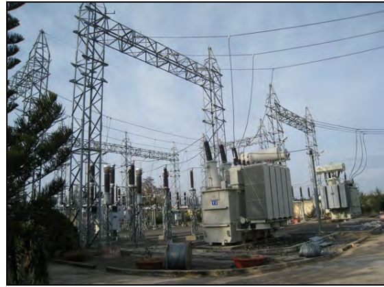
Photo 4: Phan Ri substation
