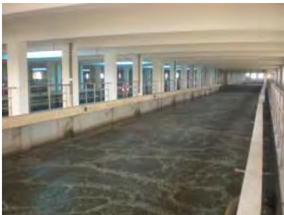
Fig. 2 Aeration tank(Hangzhou Sewage Treatment Plant)
