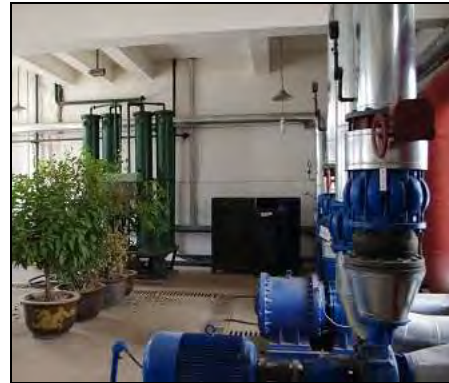
Fig.5 Heat Provision Project Central Heat Provision Facility
