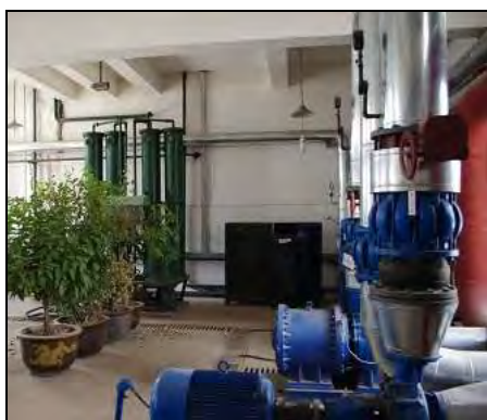
Fig. 6 Interior of a Heat Exchange Station in the City
