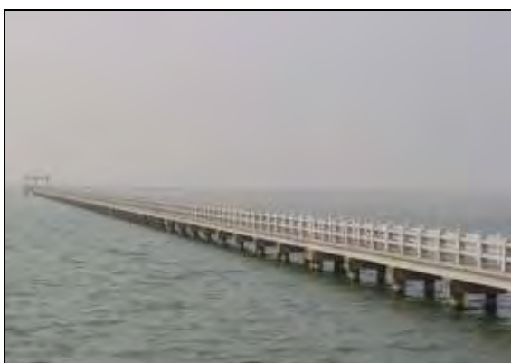
Fig.6 Water Intake at Lake Tai Shore
