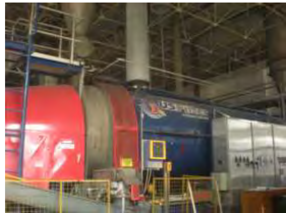
Fig. 14 Sludge dryer (Xianyanglu Sewage Treatment Plant)
