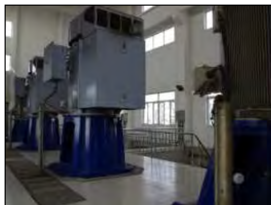
Fig.7 Intake Pumping Station
