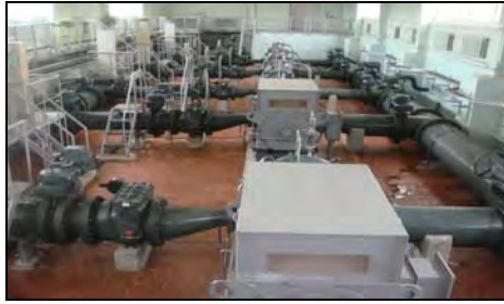
Transmission pump at upper source
