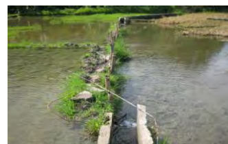
Figure 4: Partly damaged line canal
