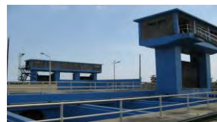
Developed pumping station in the project
