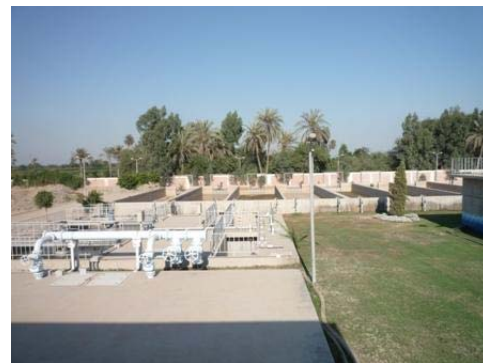
Drainage and Sludge Tanks
