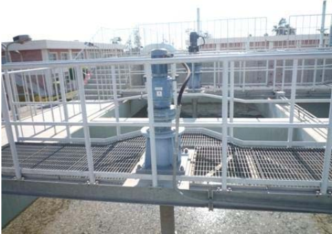
Flocculator (the blue equipment in the middle)
