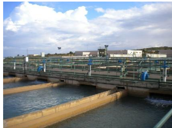
Tamri Water Purification Plant
