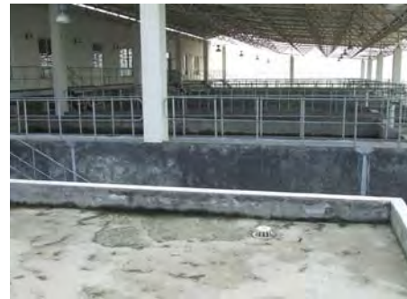
Water purification plant (Plant C)
