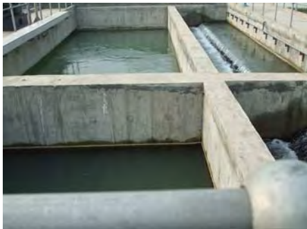
Water purification plant (Plant C)
