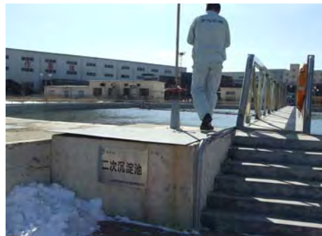
Lushunkou Wastewater Treatment Plant
