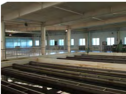
Zhuanghe Water Treatment Plant
