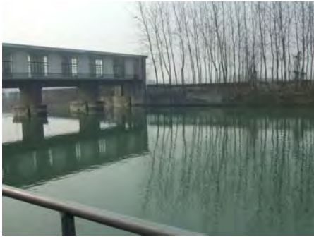
Water intake point
