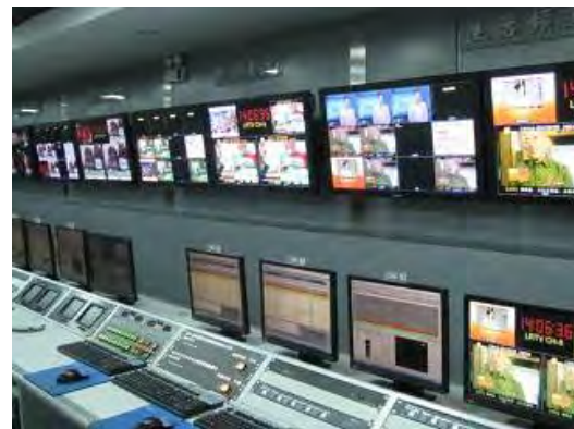
New Equipments Provided Under the Project
