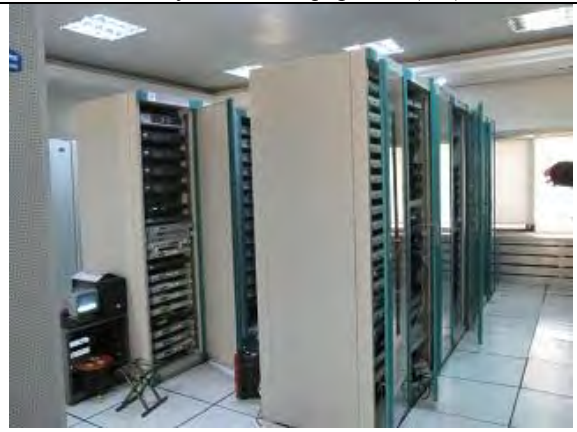
Photograph 4 Newly installed equipment (LRTTBC)
