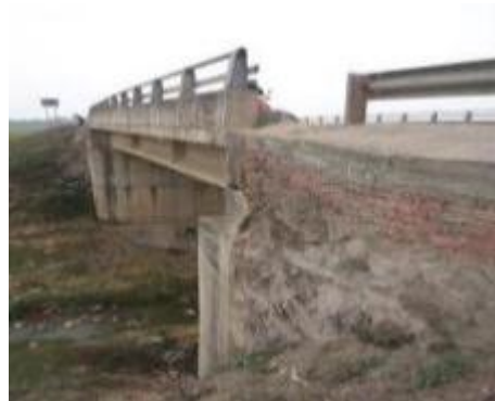
Fig. 4: Condition of the temporary
