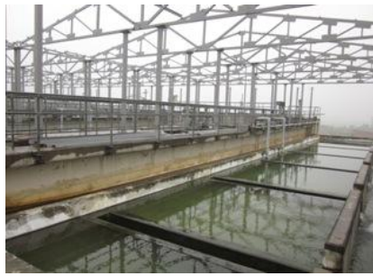
Fig. 3: Water Purification Plant
