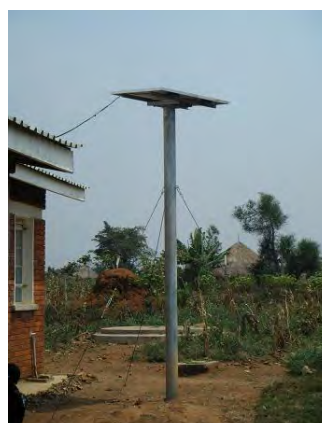
Photo: Solar system for lighting (Banda HC- III)
