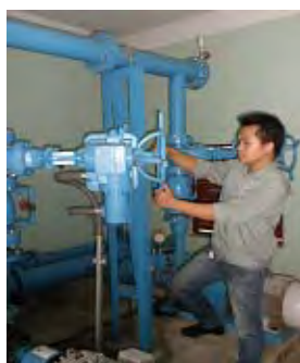
Distribution Pump (Hoa Thuong, Thai Nguyen)
