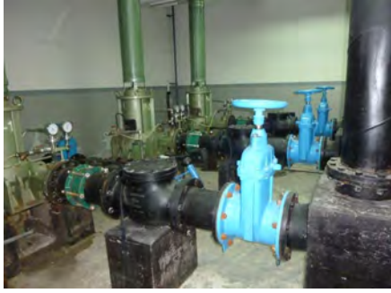
Figure 6: Booster (relay) Pump Station (Sanur Area)
