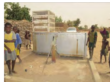
Iron-removal equipment installed along with a borehole with a hand pump (Woroyesso village in Mopti)
