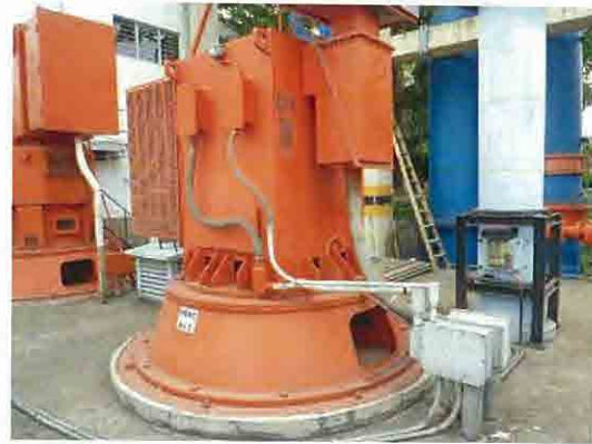
Photograph 2 Water Supply Pump (funded by the yen loan)
