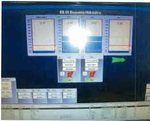
Photo 1 Monitoring the Pump Facilities
