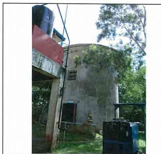
Nabaoy Intake Plant
