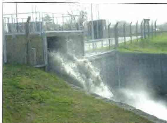
Pump Station No. 9
