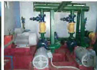
Pinaungon Pumping Station
